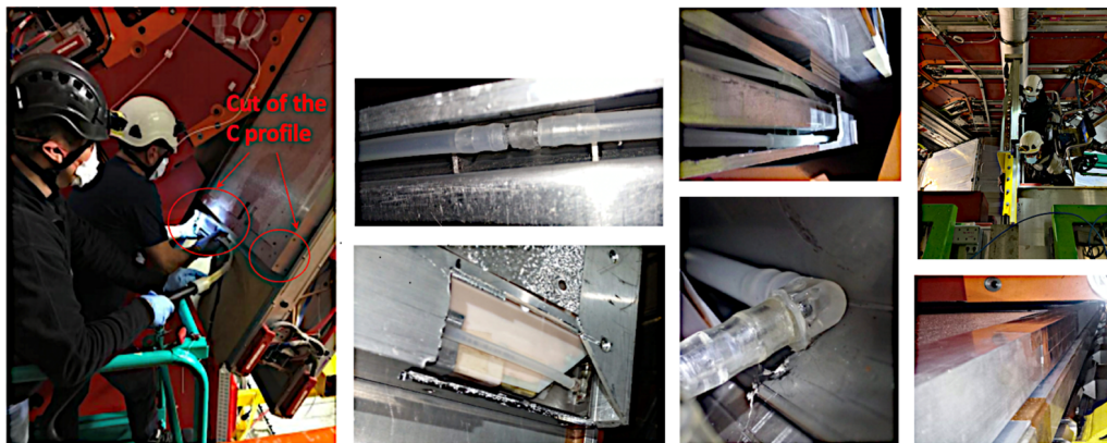
Figure 70. Photographs illustrating the gas-leak repair procedures. Left: scientists working on the repair procedure. Middle left: access to broken component. Middle right: repairing of components. Right: closing and validation.
