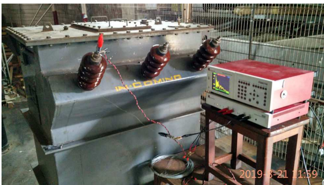
Fig. 9 Experimental set up to measure DPI on 13.8 kV winding of 11/13.8 kV, two-winding transformer with a center-tap
